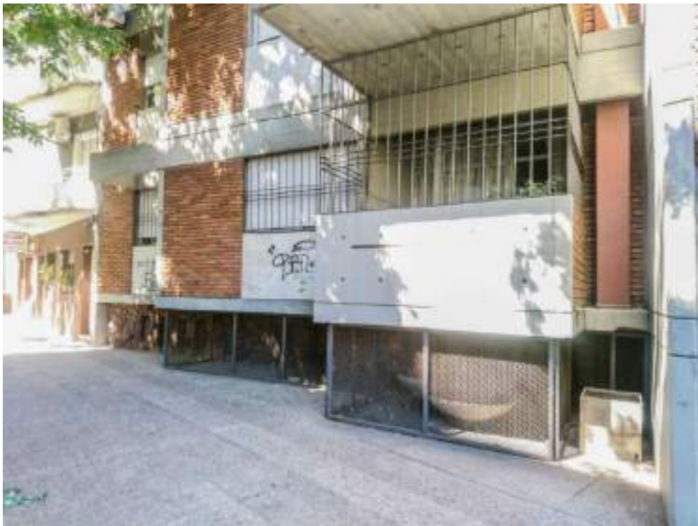
Figure 4: Example of fences and flowerpots covering possible shelters
